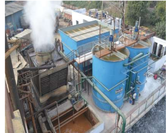
Industrial ETP Plant
