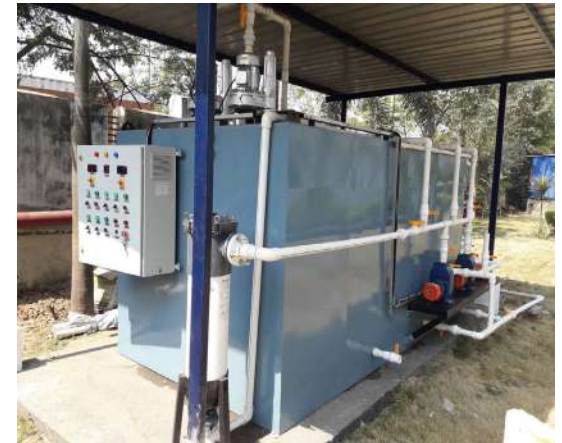
MBR STP Plant
