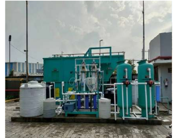
MBBR STP Plant
