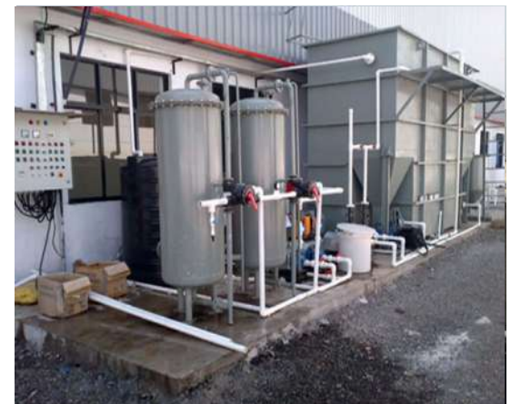
SBR STP Plant
