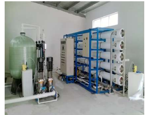
Seawater Desalination RO Plant
